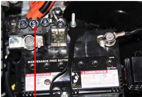
DC to DC Converter Cable Connection
